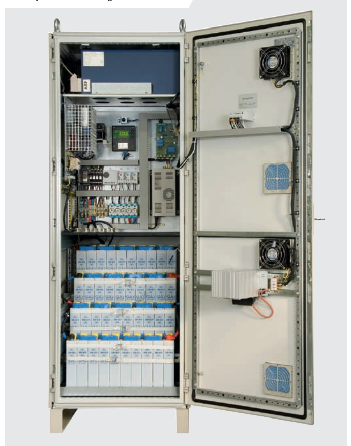
UPS system with integrated batteries
