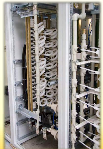
Image courtesy of CKD Elektrotechnika
